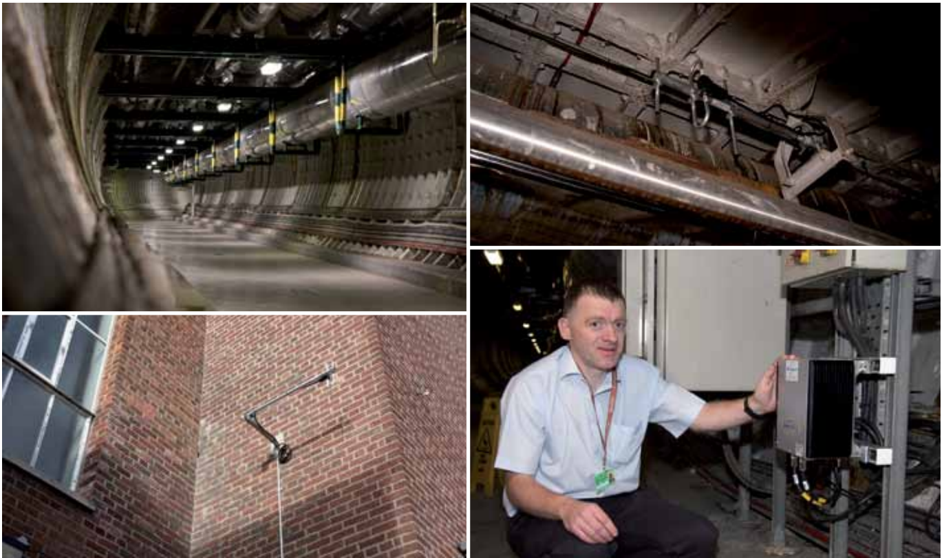
Clockwise from top left: the 'hot tunnel', built to carry steam-pipes beneath a main road which bisects the brewery site, which was one of the few areas not reached by the UHF Nexedge signal; an antenna installed within the tunnel as part of a coverage reinforcement system provided by PMR supplier BP Multipage; Dave Gerachty, service manager for BP Multipage, with the tunnel booster he installed, a bidirectional amplifier by the French manufacturer ETSA; and, on a wall outside, the pickup antenna which feeds the tunnel amplifier
